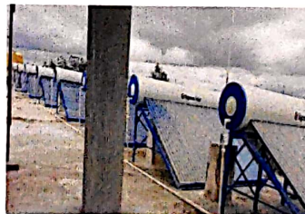
SOLAR WATER HEATERS AT GIRL'S HOSTEL
